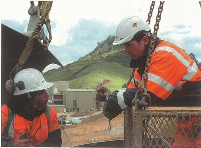
Brian Perry Civil project manager Jason Giacopazzi and his team prepare to gain access to the ventilation shaft
